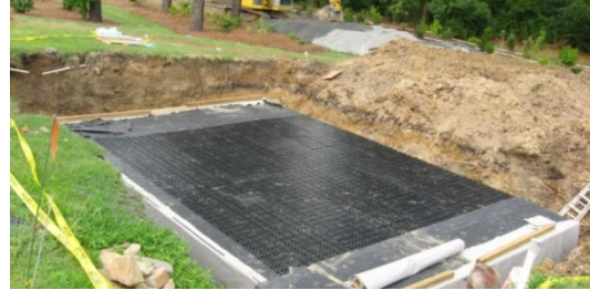
Subsurface Detention Gallery
