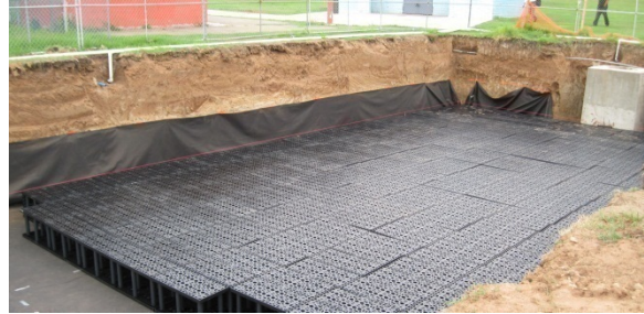
Subsurface Infiltration Gallery
