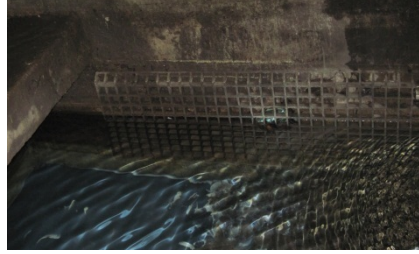
Low-Flow Diversion Dam and Inlet in a Storm Drain
